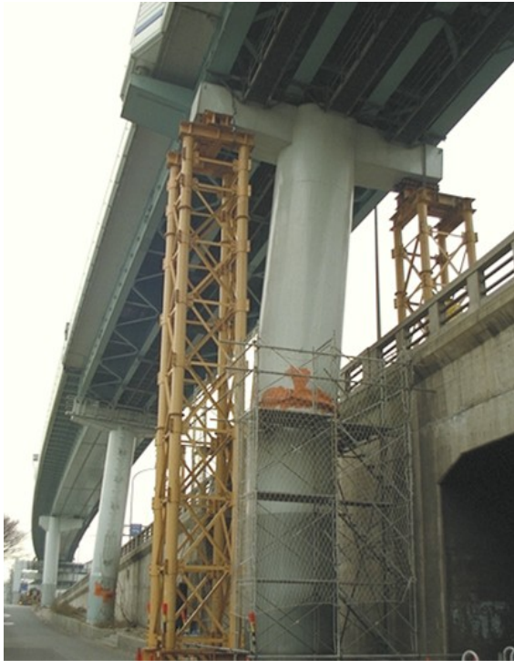
Local buckling in steel piers
