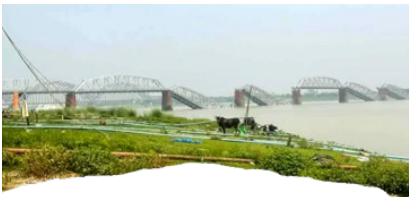
Unseating damage, Ava bridge 2025 Myanmar earthquake
