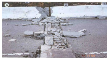
Pounding damage, Wuxi bridge 1999 Taiwan ChiChi Earthquake
