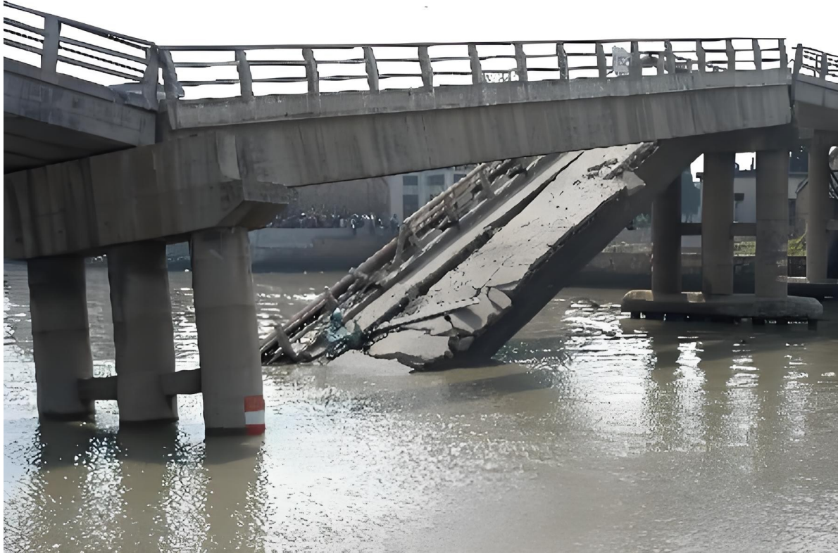
Girder Falling / Nonstructural elements damage
